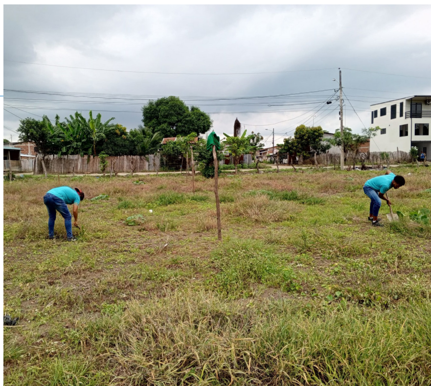
Two young volunteers help clear the land for construction. Soon, this lot will be home to a new church building with classrooms, restrooms, a kitchen and dining room.
